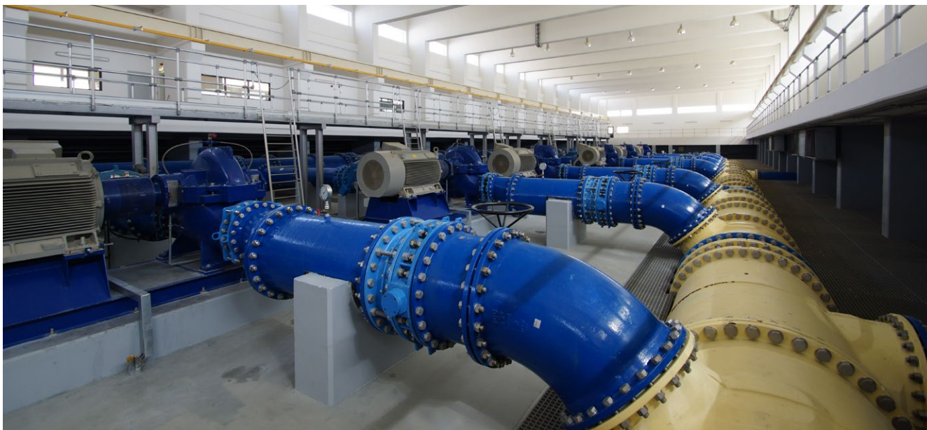
Sohar. Aspiracion Intermediate Pumping Station (Omán).
